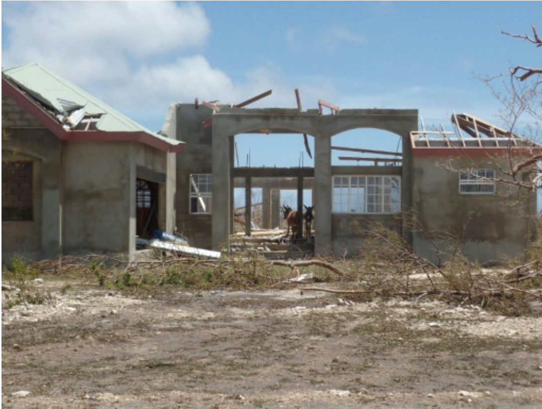
Houses in Codrington, Antigua and Barbuda, devastated by Hurricane Irma
