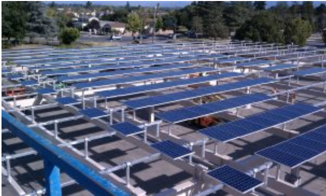
Solar array at De Anza College in San Francisco. Credit: Darin Dingler
