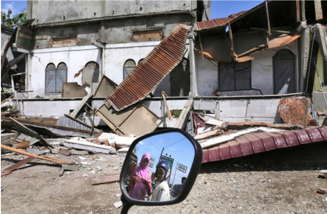
Women are reflected in a motorbike's mirror as they access the damaged building after an earthquake in Pidie Jaya, Aceh province, Indonesia, Wednesday, Dec. 7, 2016. A strong undersea earthquake rocked Indonesia's Aceh province early on Wednesday, killing a number of people and causing dozens of buildings to collapse. (AP Photo/Heri Juanda)
