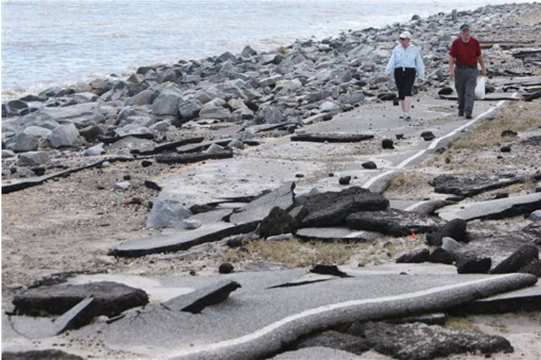
Lee and Gary Moulton walk from their home along what is left of a road that was destroyed by Hurricane Hermine in the Alligator Point community of Franklin County, Fla., Friday, Sept. 2, 2016. (Andrew Wardlow/News Herald via AP)
