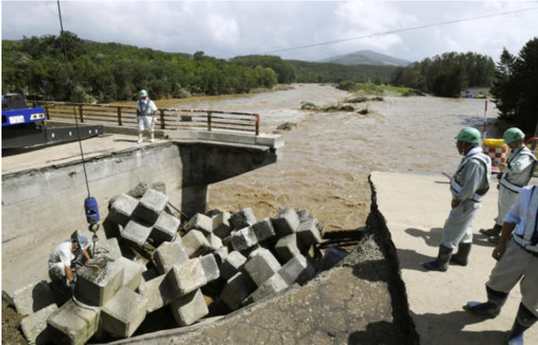
Workers repair a flood damaged bridge over the Sorachi river in Minami-furano, the northern island of Hokkaido, Japan, Wednesday, Aug. 31, 2016. Typhoon Lionrock dumped heavy rains on the areas in northern Japan. (Daisuke Suzuki/Kyodo News via AP)
