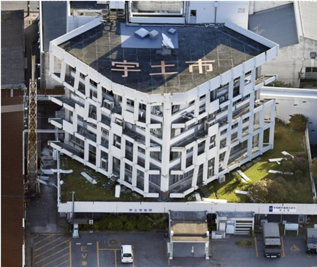
Exterior wall of the city hall fall off after the earthquake in Uto, Kumamoto prefecture, southern Japan Saturday, April 16, 2016. A powerful earthquake struck southern Japan early Saturday, barely 24 hours after a smaller quake hit the same region. (Muneyuki Tomari/Kyodo News via AP)
