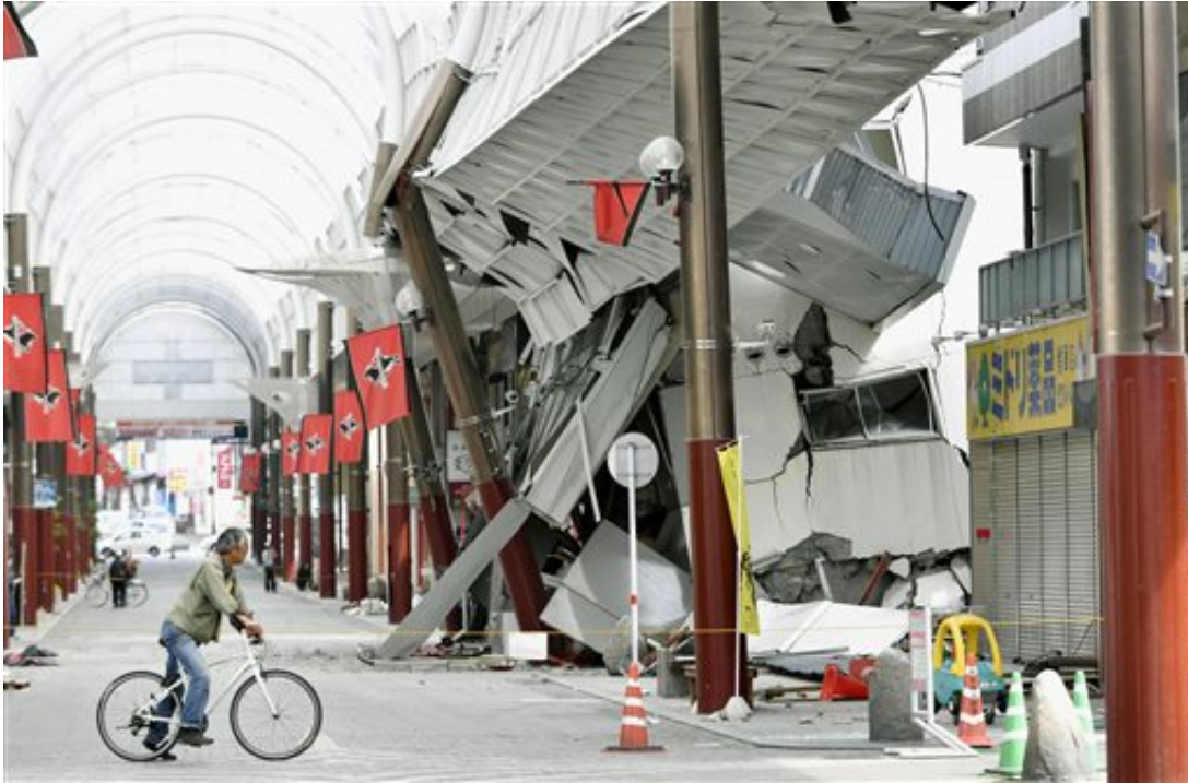
A cyclist looks at a shopping arcade destroyed by the earthquake in Kumamoto city, southern Japan Saturday, April 16, 2016. A powerful earthquake struck southern Japan early Saturday, barely 24 hours after a smaller quake hit the same region. (Kyodo News via AP)
