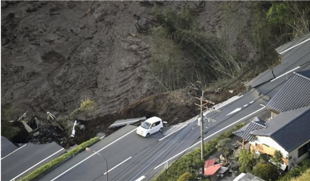
A car sits on a road collapsed by an earthquake in Minamiaso, Kumamoto prefecture, southern Japan Saturday, April 16, 2016. A powerful earthquake struck southern Japan early Saturday, barely 24 hours after a smaller quake hit the same region. (Muneyuki Tomari/Kyodo News via AP)
