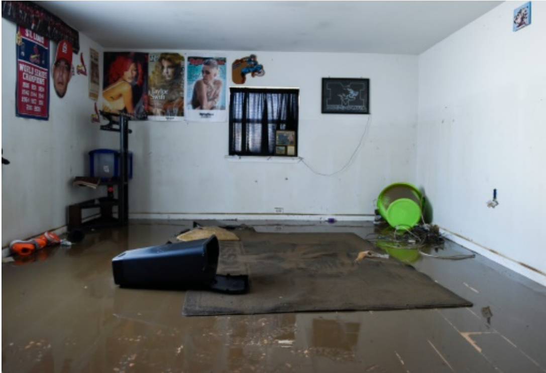
Debris and water covers a floor in the home of Debbie and Benton Kelly in Pacific, Missouri on January 1, 2016
