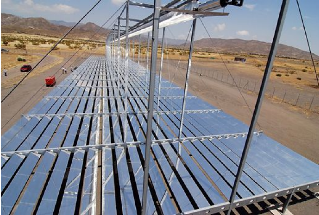
Linear Fresnel collector demo MAN installed at the Solar Platform in Almería (PSA). Credit: PSA
