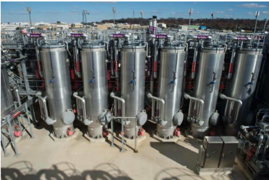
The hydrolysis wastewater treatment center is seen at DC Water's Blue Plains plant in Washington, DC
