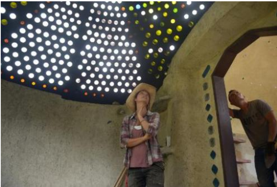
Alexandra Posada (C) pictured with a glass bottle skylight during the building of her house in Choachi, Cundinamarca, Colombia on March 16, 2015
