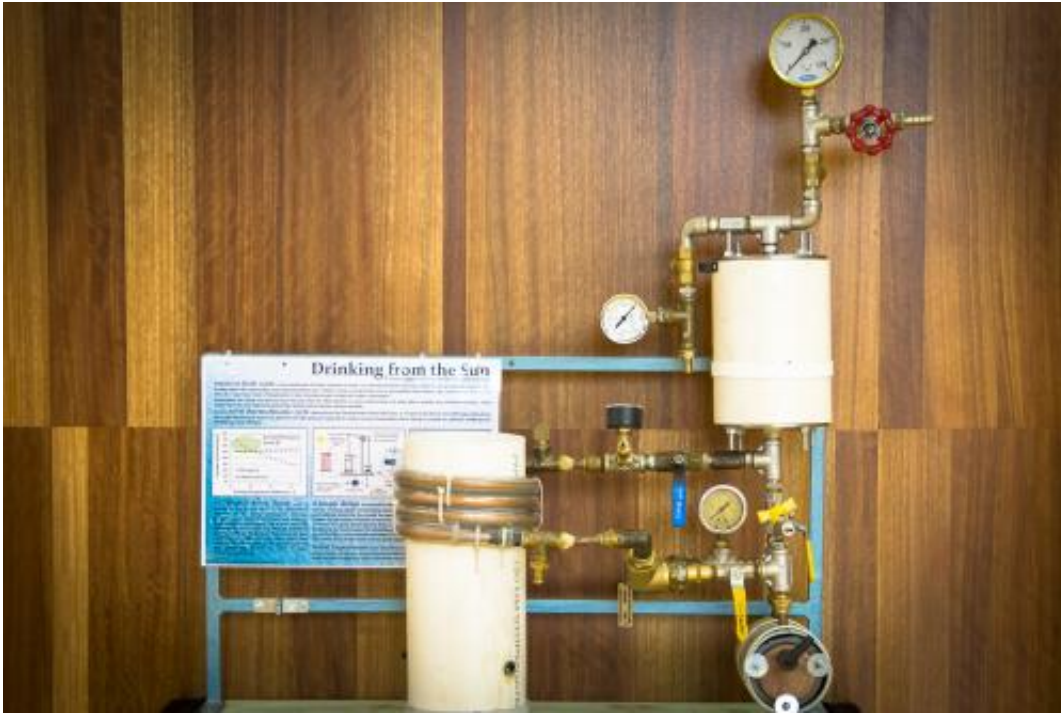
Thermal Water Pump. Credit: RMIT University
