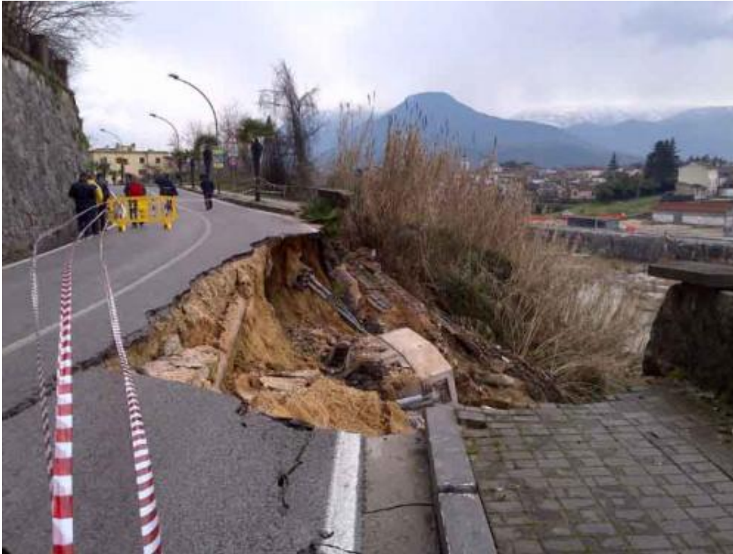
Landslide area. Credit: NHAZCA
