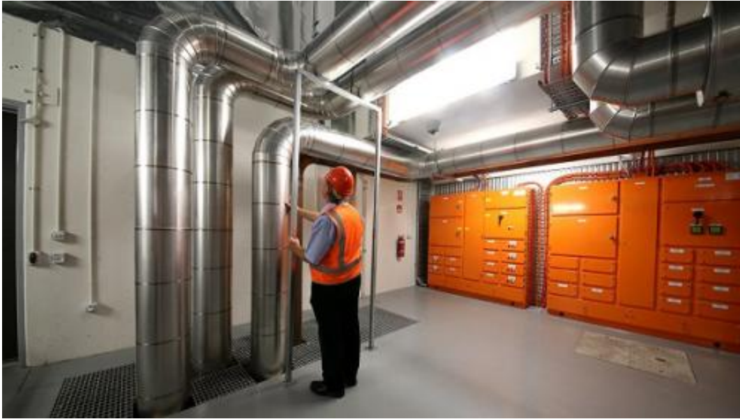
The Pawsey Centre plant room that houses the cooling and electrical systems. Credit: CSIRO
