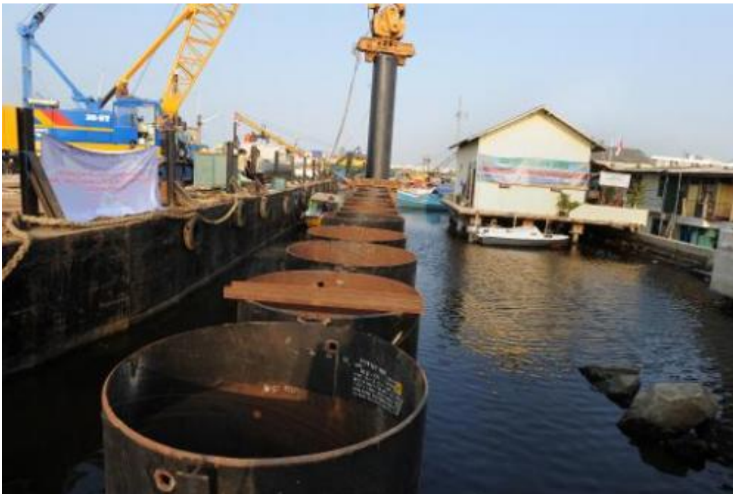
A wall of giant iron reinforcement pipes is installed during the construction of the Jakarta sea wall, October 9, 2014
