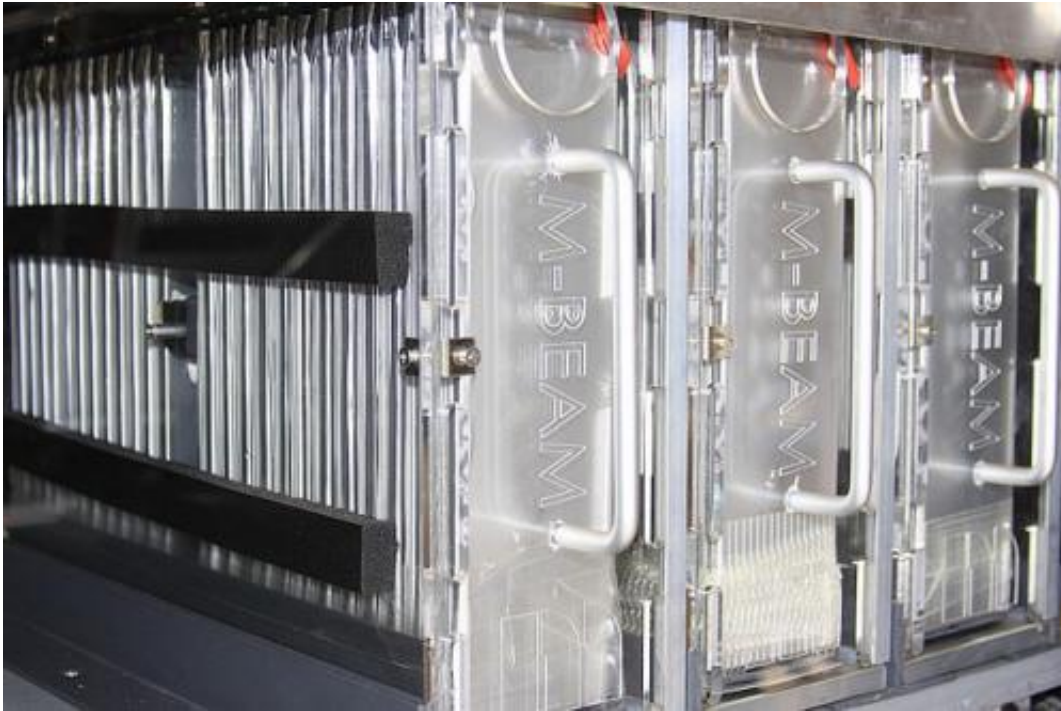
Close-up of the battery modules.
