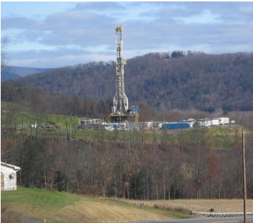
Derrick and platform of drilling gas wells in Marcellus Shale - Pennsylvania. Credit: Wikipedia/ CC BY-SA 3.0
