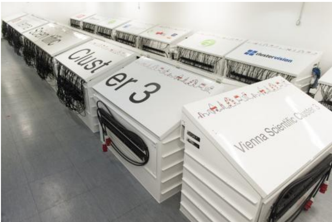
A view of the Server Room of VSC
