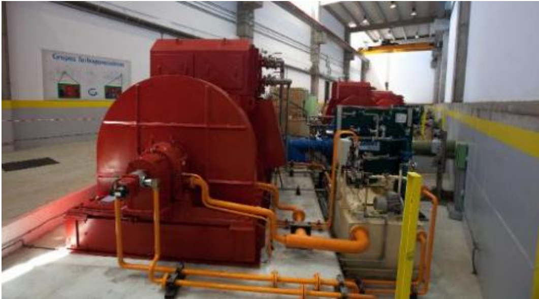
A Turbogenerator set (L) and a lubrication (blue) at the Gorona power station on El Hierro island on March 28, 2014
