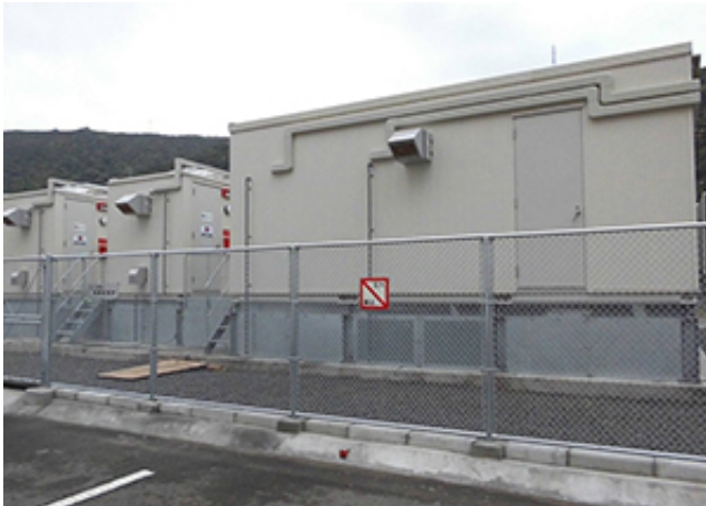
Lithium-ion battery energy storage system for Tatsugo Substation.
