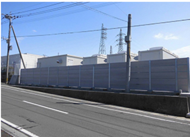
Lithium-ion battery energy storage system for Naka-Tane Substation.
