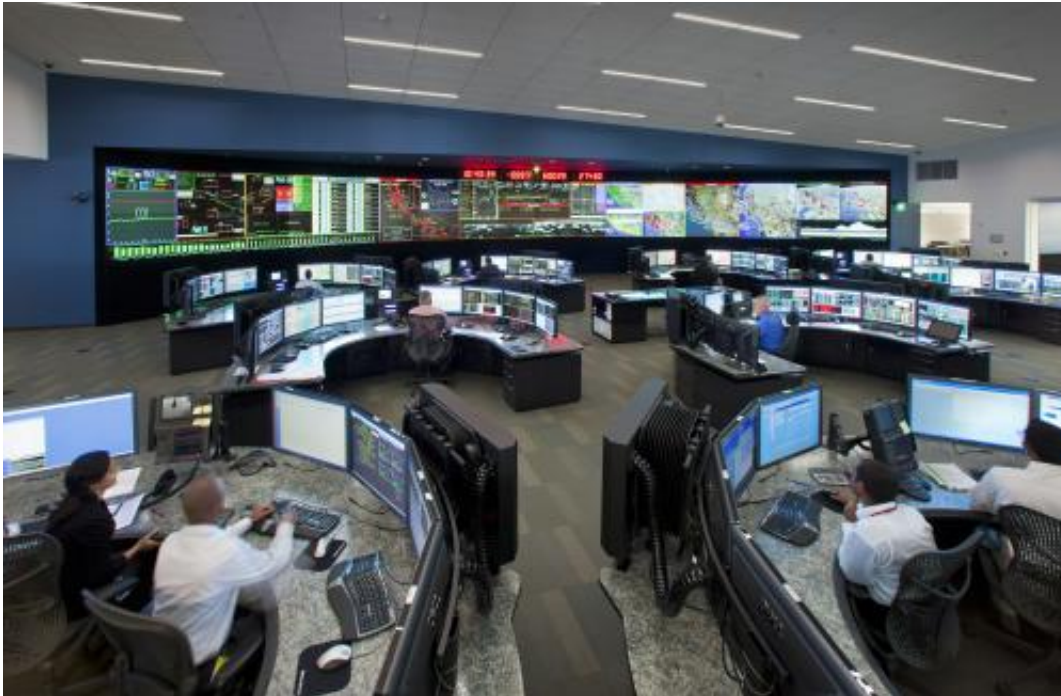
Control room at California Independent System Operator.
