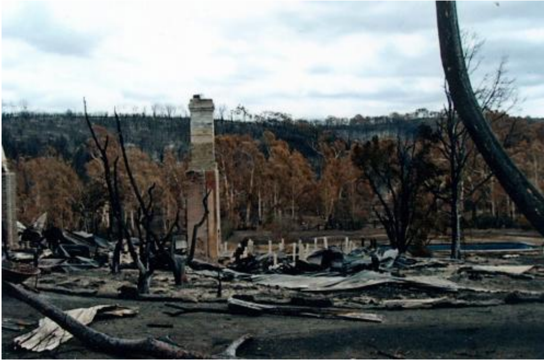
Damage caused by the Back Saturday fires. Credit: AAP Image/Supreme Court Victoria
