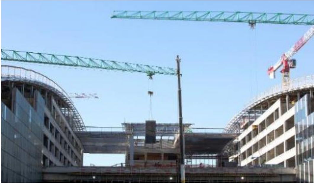
A view of the new NATO headquarters under construction in Brussels on November 13, 2013
