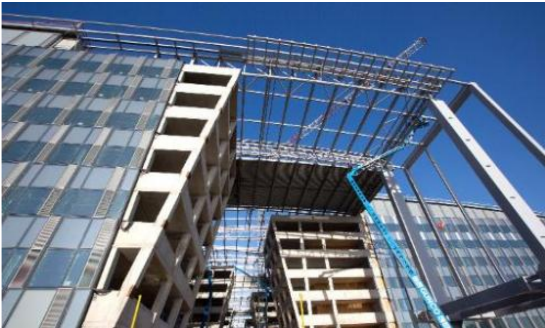
A view of the new NATO headquarters under construction in Brussels on November 13, 2013
