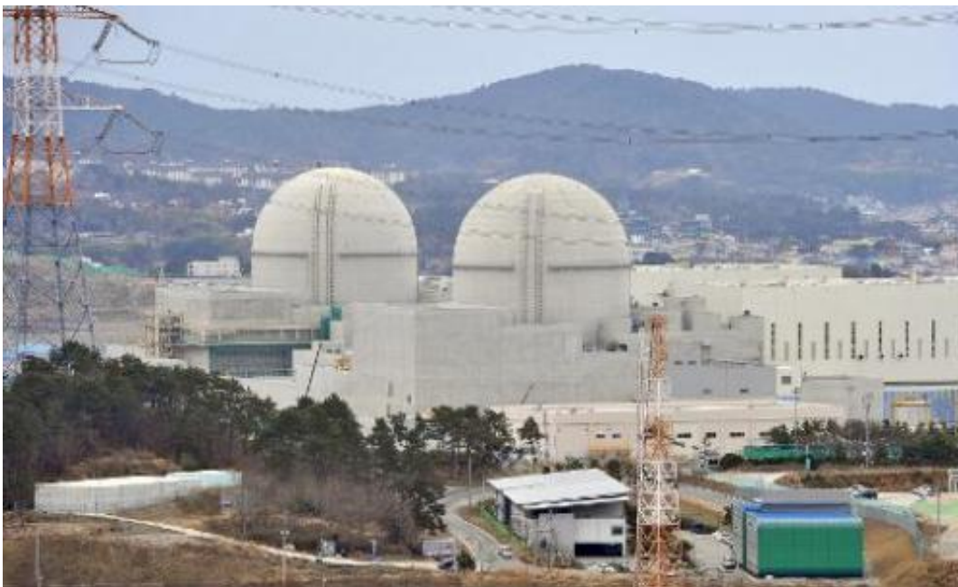
The Shin-Gori 3 and 4 reactors under construction in Gori near Busan on February 5, 2013
