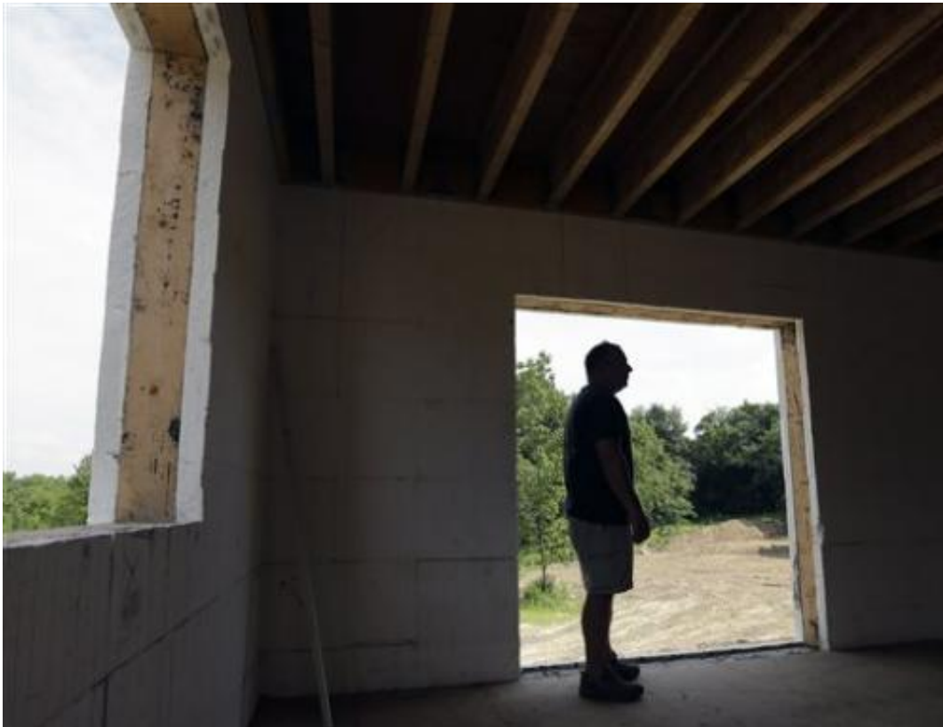
Gil Lobell stands in his zero net energy home that is under construction at The Preserve at Mountain Vista on Tuesday, July 9, 2013, in New Paltz, N.Y. (AP Photo/Mike Groll)
