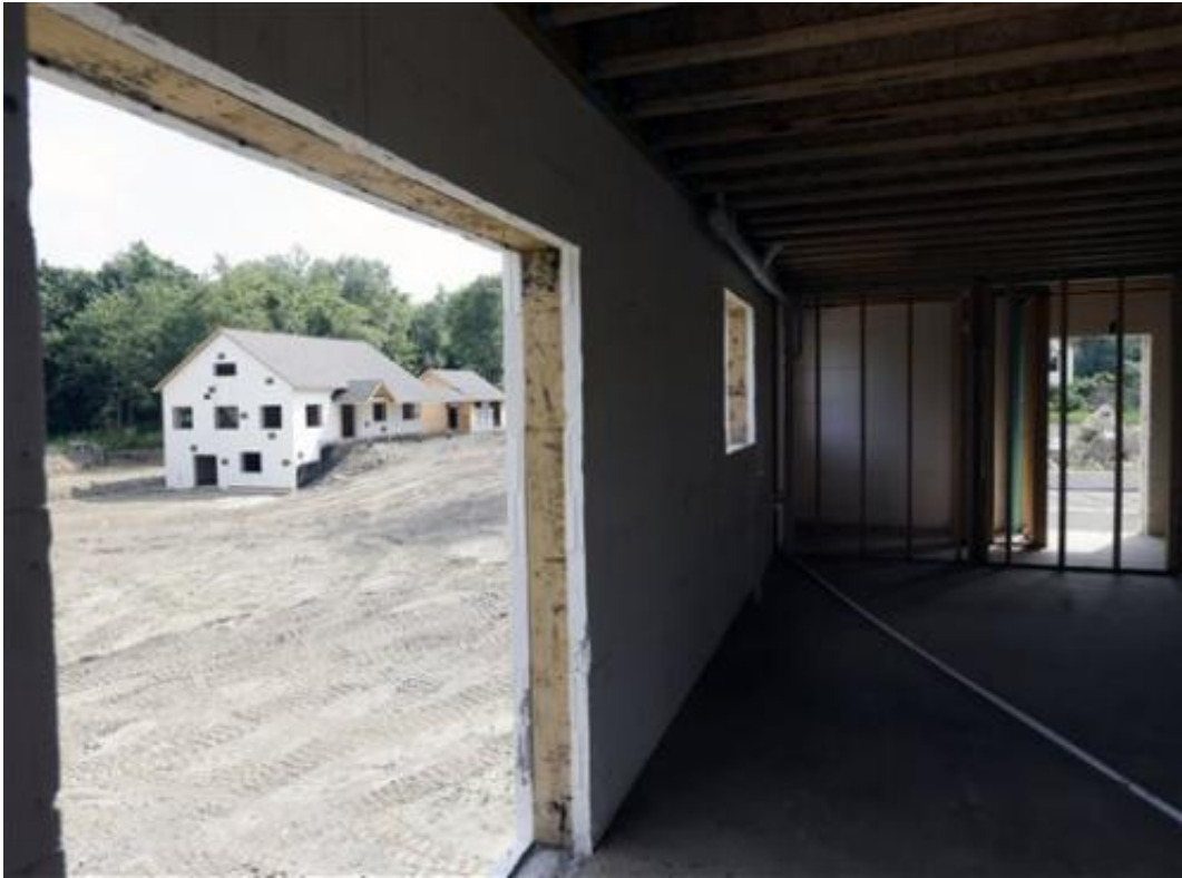
A zero net energy home under construction is seen from the interior of another at The Preserve at Mountain Vista on Tuesday, July 9, 2013, in New Paltz, N.Y. (AP Photo/Mike Groll)
