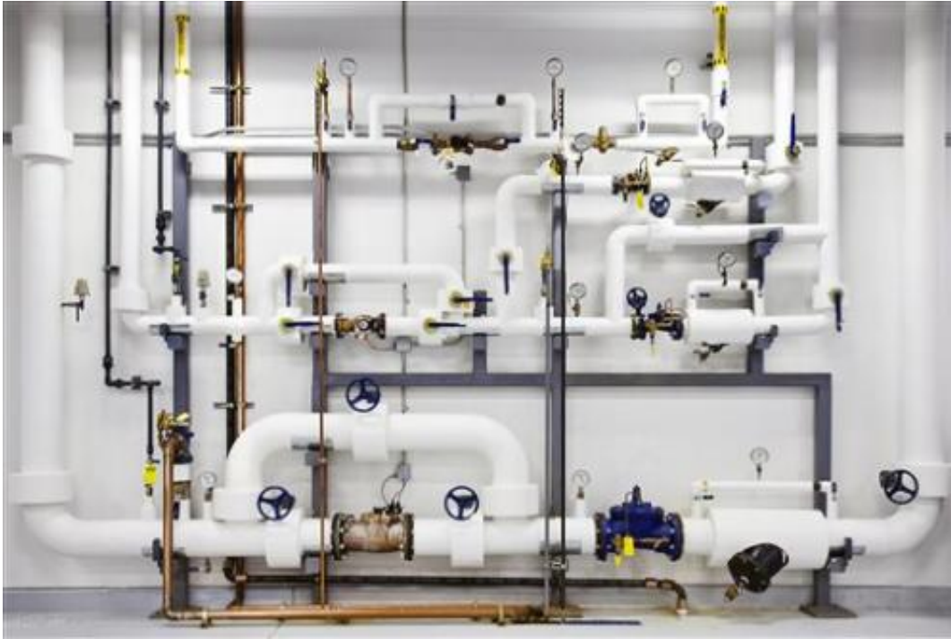
This undated photo made available by Google shows pipes with highly pressurized water at Google's data center in Douglass County, Ga. (AP Photo/Google, Connie Zhou)
