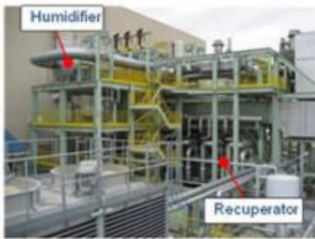
Fig. 1 Full view of the 40MW test facility
