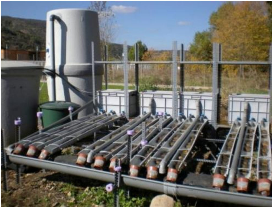
The Mesocosmos Sostaqua, an infrastructure located at the Balsareny water-treatment plan. Credit: FEM Research Group-UB
