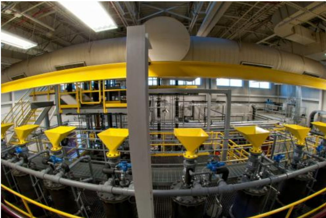
Wood to sugar hydrolysis units in Viridia's pilot plant in Danville, VA.
