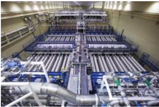
Laser Bay 2, one of NIF's two laser bays
