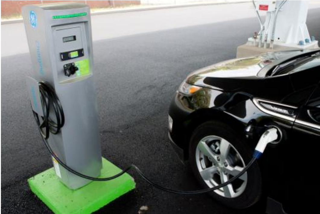
GE EV Solar Carport in Plainville, CT
