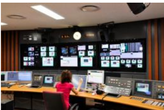
Master Control Equipment installed at Fuji TV
