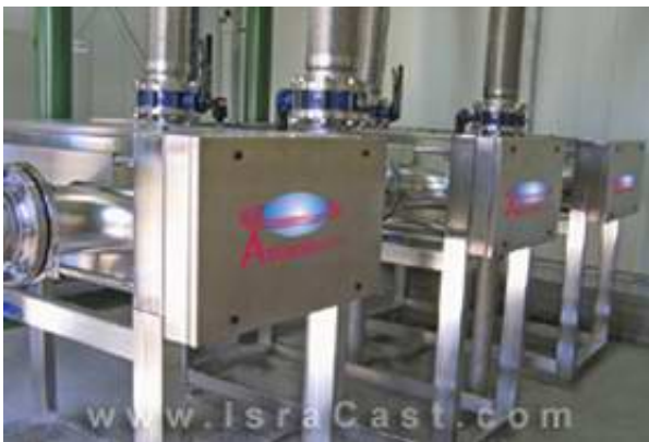
Three UV-JETs, installed at Tnuva&acutes new plant
